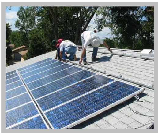
Workers install a solar system on a zero-energy home. The system has both photovoltaics and solar thermal collectors and will provide enough electricity and hot water to meet all the occupants' needs. (Photo—Pete Beverly)
